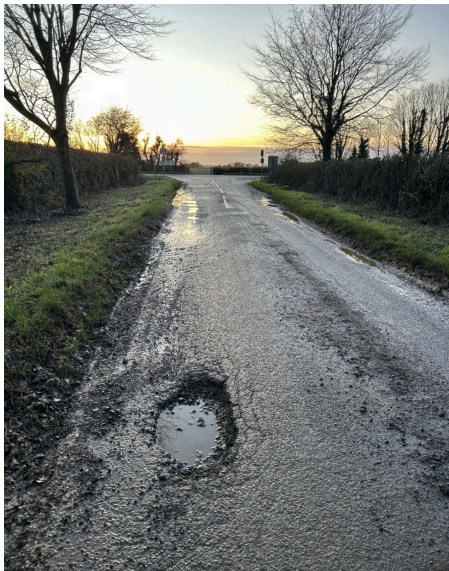
Potholes, Second Turn.
